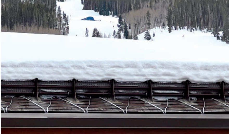
Zigzag pattern of heat trace cables below the snow fence at the eaves. PHOTO COURTESY OF FLO-TRACE
