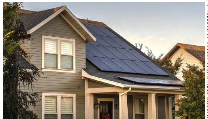
ALL PHOTOS COURTESY OF BELMONT SOLAR, GORDONVILLE, PENNSYLVANIA.
