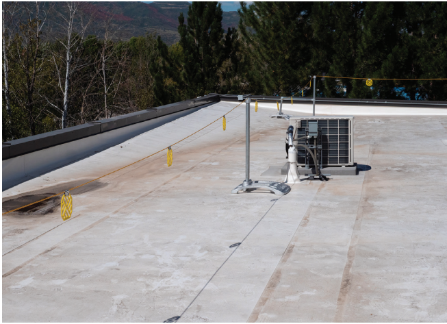
A warning-line fall protection system. Courtesy of Diversified Fall Protection.
