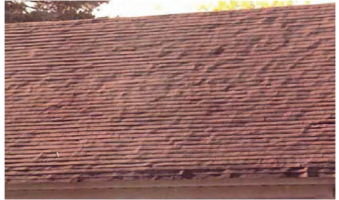
Example of buckled shingles. Photo courtesy of GAF.
