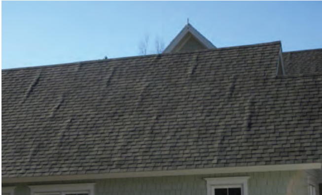
Example of buckled shingles. Photo courtesy of CertainTeed.
