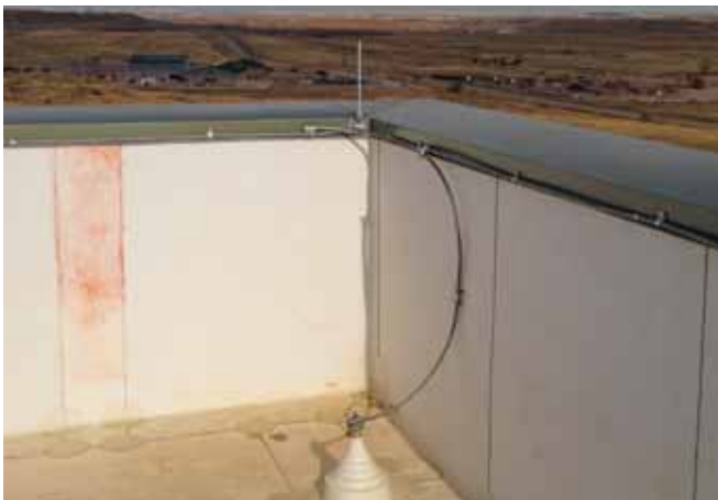
Rooftop lightning protection components correctly installed along the inside of the parapet.
