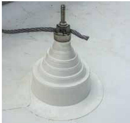
This is a properly installed lightning protection system through-roof penetration.
