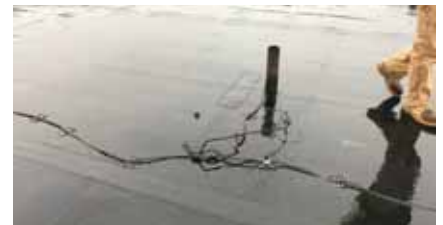
All sorts of problems become possible when lightning protection cables are not properly fastened.
