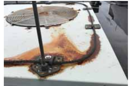
Anyone working with a lightning protection system must be aware of the problems caused by the contact of dissimilar metals, like copper components on an aluminum air conditioning unit.
