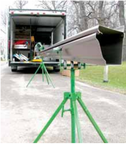
Leafaway Gutters being manufactured on site with an Eastside Machine portable roll former. ALL NEW GUTTER SERVICE PHOTO
