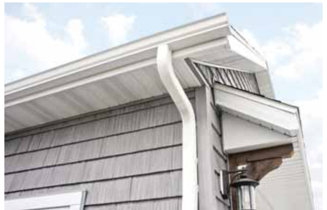
An All New Gutter installation featuring a complete rain carrying system in traditional white. ALL NEW GUTTER SERVICE PHOTO
