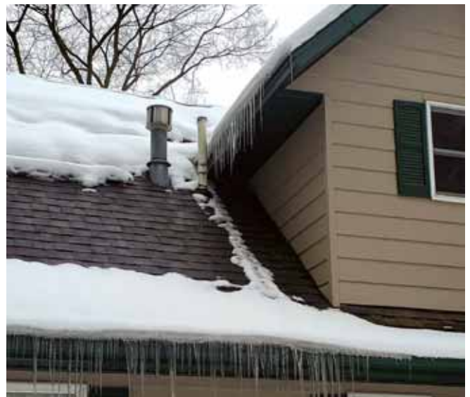
The lack of snow in the roof plain shows where heat is transferring from the conditioned living space to the attic, indicating inadequate insulation and/or inadequate ventilation. PHOTO COURTESY OF TIM CHAPIN, YOUR SAFE AND HEALTHY HOME, AKRON, OHIO.
