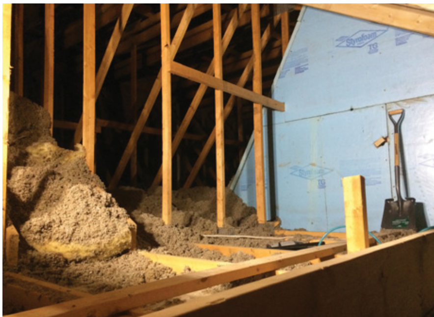
As loose, blown-in insulation settles, it becomes less effective. PHOTO BY JACOB PRATER.
