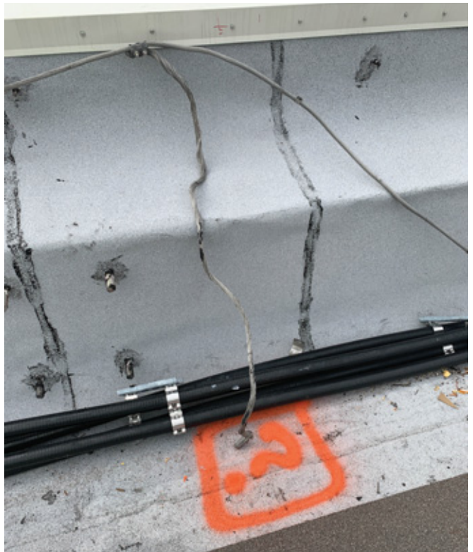
Integrating lightning protection systems with roofing system components often leads to questions surrounding penetrations and sequencing.
