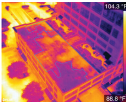
Areas highlighted in blue are suspected to be wet. PHOTO COURTESY OF STRUCTURA VIEW
