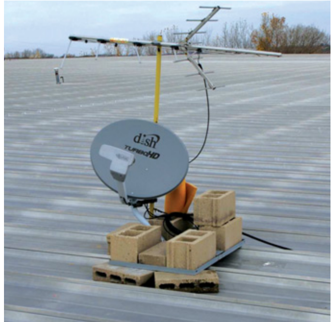
The WRONG way: Ballasted systems require structural analysis for resulting point loads; the alkali in cementitious ballast corrode coated steel roofing.
