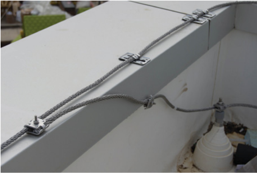
Bonding connects the LPS to other internally grounded metallic systems on the roof, such as air conditioning units, vent stacks, and other components, to create a path for the lightning current.
