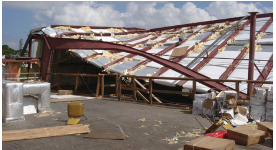
Tornado damage caused during Hurricane Wilma. Overall damages caused by Hurricane Wilma totaled $29 billion. PHOTO COURTESY OF ROOF HUGGER, LLC.
