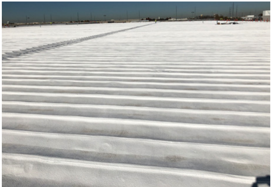
Only 300,000 square feet needed to be repaired on a one million square foot job. PHOTOS COURTESY OF POLYGLASS.
