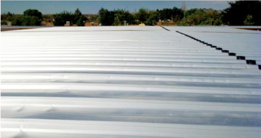
Metal panel buckling caused by improper pinning of long standing seam panels. PHOTO COURTESY OF ROOF HUGGER, LLC.
