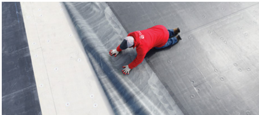
Cover boards contribute to long-term performance of commercial roofing systems.
