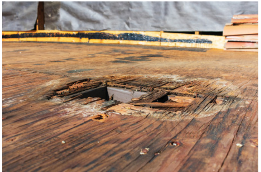
Moisture buildup in the roof assembly can result in deck deterioration.
