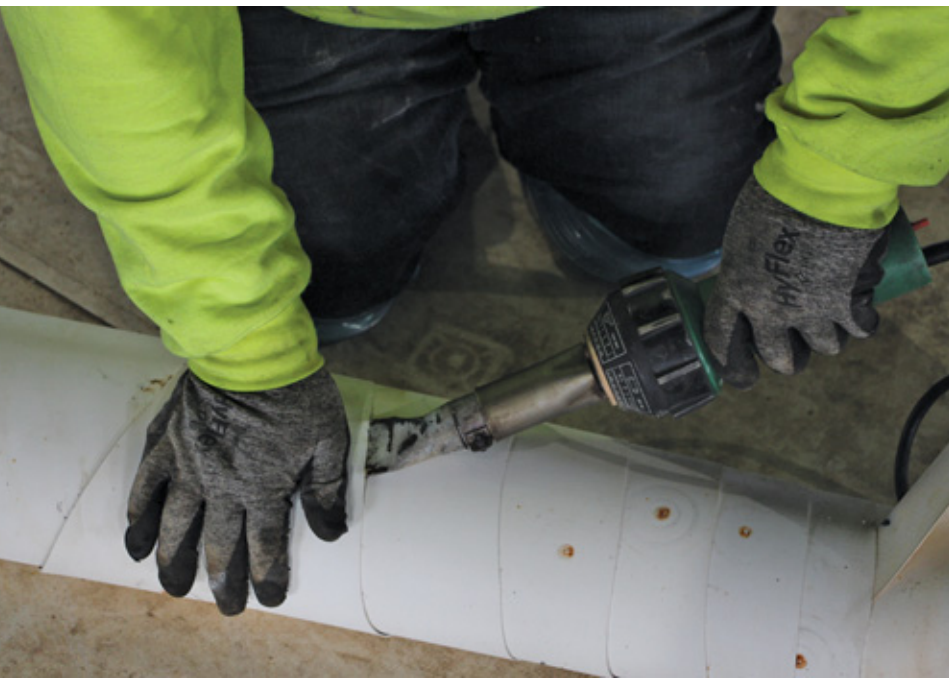
The most effective means of preparing the old membranes for transport to the recycler appears to be for them to be cut into strips of prescribed widths and lengths and tightly rolled and tack welded before leaving the job site for the recycler.
