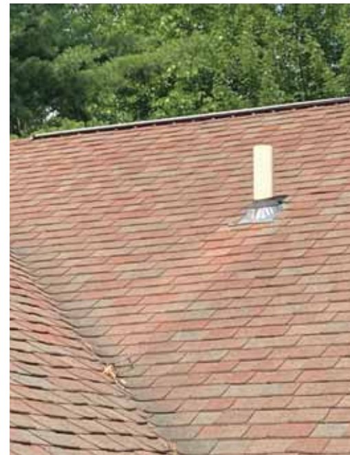
Organisms need moisture to grow. Note there is no algae growing below the pipe flashing on this roof.
