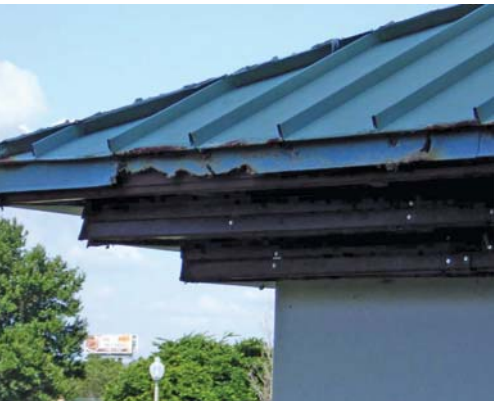
Selecting and using the wrong product in a corrosive (seaside) environment can result in premature failure of the materials. Photo courtesy of Petersen.
